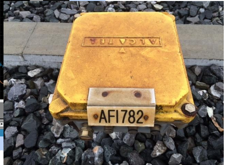
Traffic monitoring induction loop
