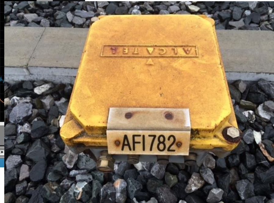
Traffic monitoring induction loop
