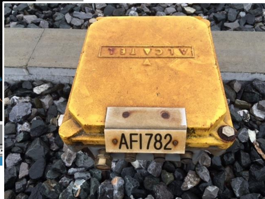
Traffic monitoring induction loop
